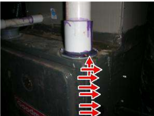
A. Picture 1 water running down furnace
