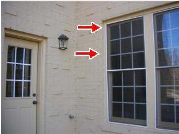
I. Picture 1 screen loose
