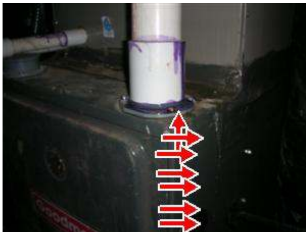
A. Picture 1 water running down furnace
